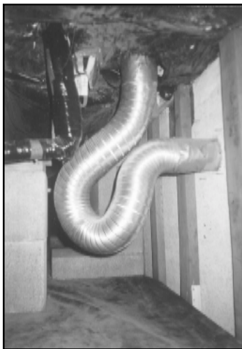
Dryer ducts are frequently installed incorrectly. This installation uses the right material (rigid flexible metal, not metal foil), but uses too much of it. Ducts should be installed with no dips or traps where water and lint can collect. This could be corrected by shortening the duct to eliminate the trap.
