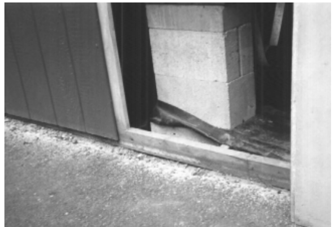
Figure 2: This skirting is made of siding material not rated for ground contact.
