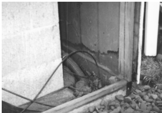
Figure 3: Just three years after installation, deterioration is visible.
