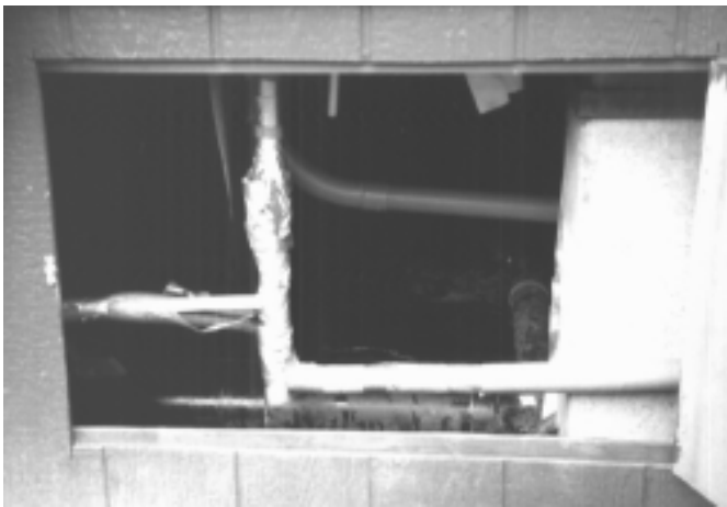
Figure 1: This access opening is the right size, but it's blocked by pipes, piers, and lines.
