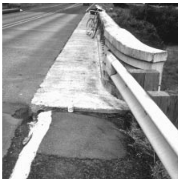
Sidewalk ramp should be raised
