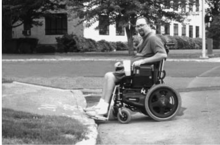
Pavement grinding project left exaggerated lip at this curb cut
