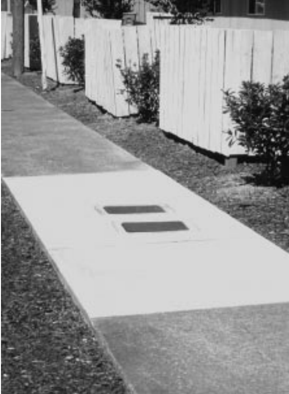
Utility cut is flush with sidewalk
