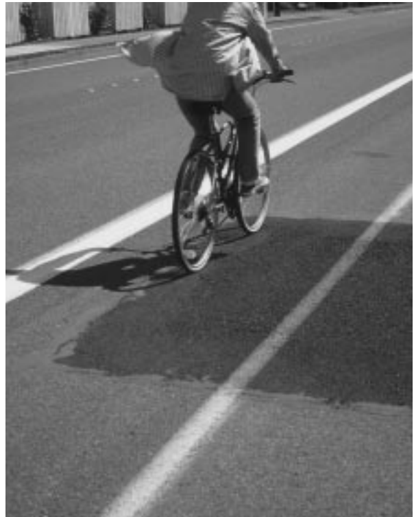
Patch extends only halfway into bike lane
