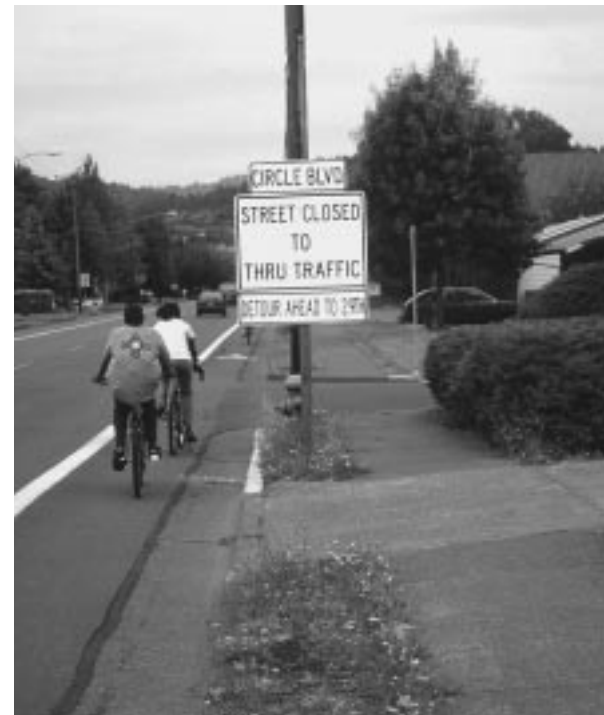
Construction signs placed out of bike lane and sidewalk
