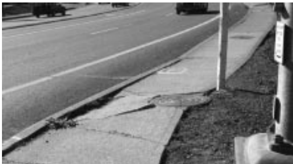
Sidewalk in disrepair
