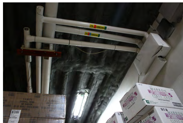
Pipes are well marked in the refrigerated warehouse.
