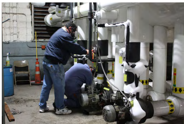
Barron oversees the restoration of an ammonia pump while wearing proper protective equipment.
