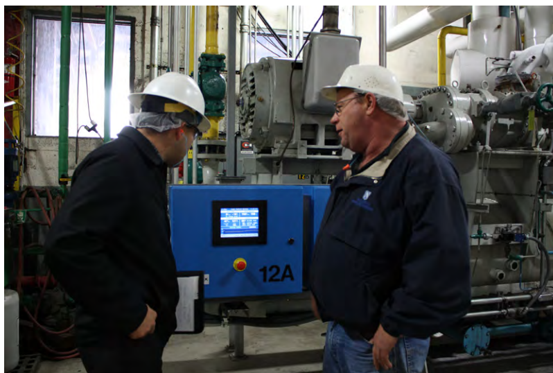
Nunez (left) and Barron review settings on a compressor control system recently installed.
