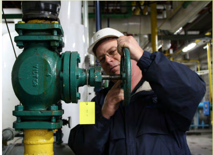
Barron takes a look at an older valve in the system.
