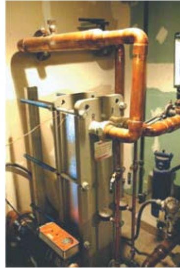
Figure 4. Photograph of the heat exchanger between the City geothermal district heating system and the brewery secondary heating loop.
