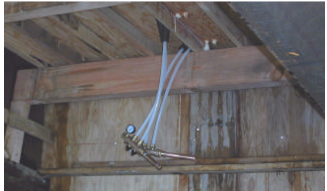
Figure 7. Manifold under the bridge deck before they are placed in boxes.
