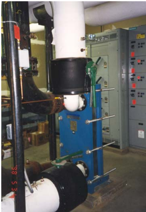
Figure 2. Photograph of one plate and frame heat exchanger at the Inn of the Seventh Mountain.
