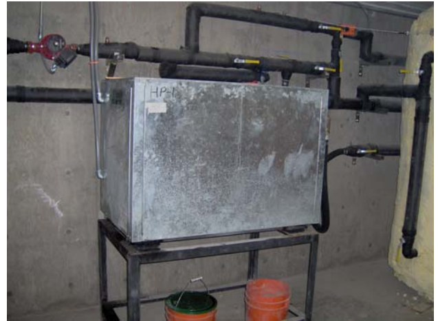
Figure 3. Photograph of the 15 ton water-water heat pump serving the entire building. Note the storage tank on the right.
