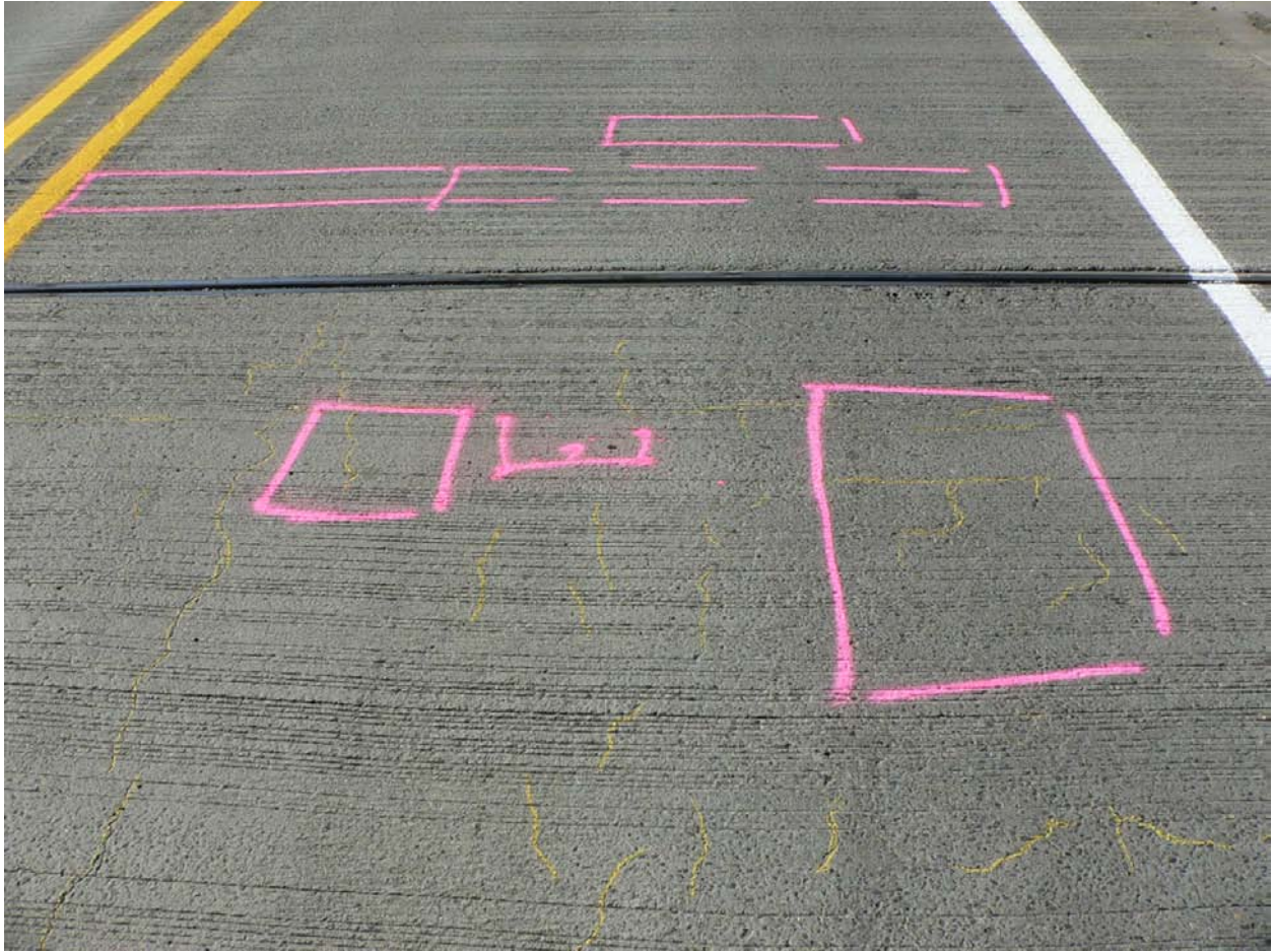
Figure 2.1: Highlighted cracks and marked delaminations.
