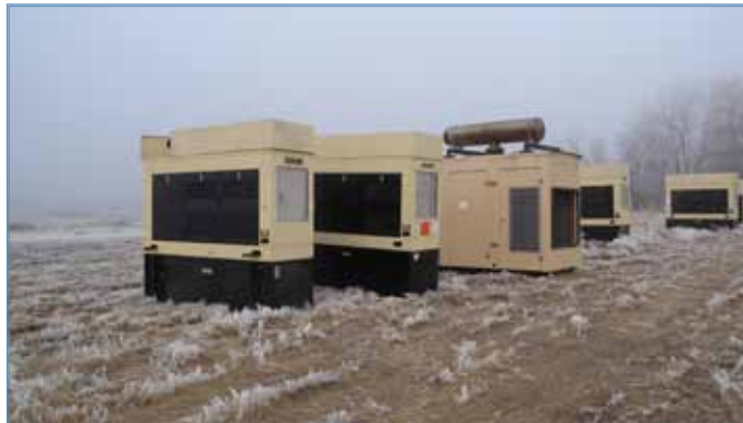
These CSEPP emergency generators have been prepared for shipment to new locations at tribal, public safety, city and county facilities throughout Oregon.
