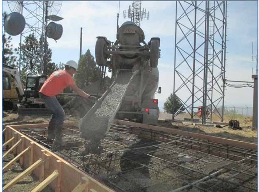
An employee from Summit Solutions/ADK guides the concrete chute and works to prepare the foundation for a new shelter on Grizzly Mountain in Crook County.
