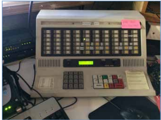
The 30-year-old Zetron console at the Oregon State Fairgrounds is used by Oregon State Police dispatchers during the run of the State Fair. Next year, the Zetron will be replaced by a new digital console with multi-channel capabilities.
