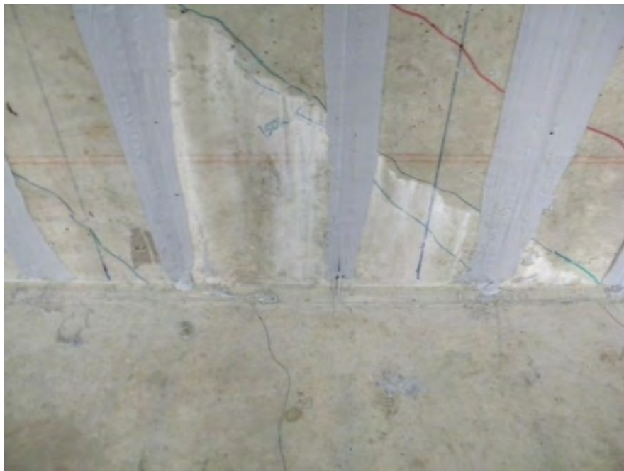
Figure 6.14: Specimen IT.7.22.6.FTG typical efflorescence
