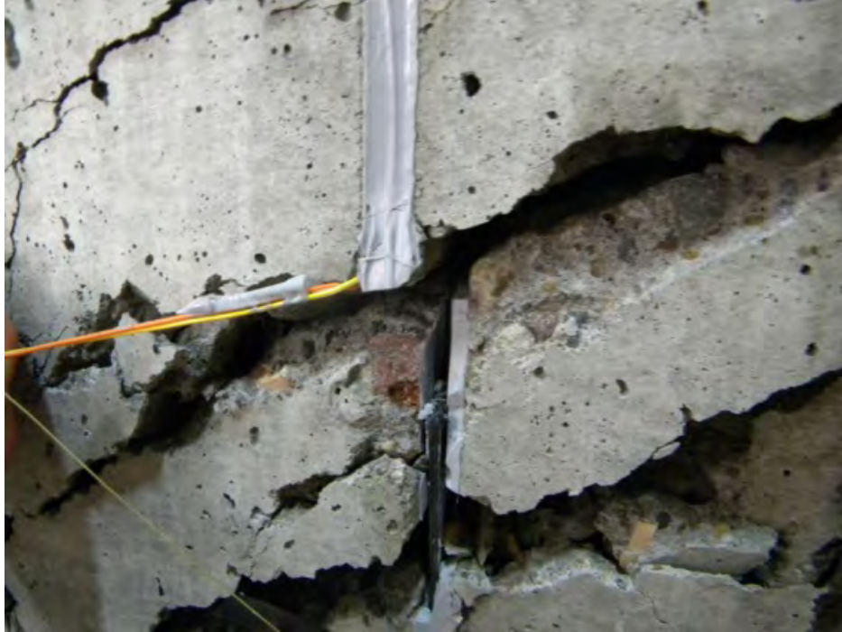
Figure 6.17: IT.7.22.6.FT/FTG CFRP rupture
