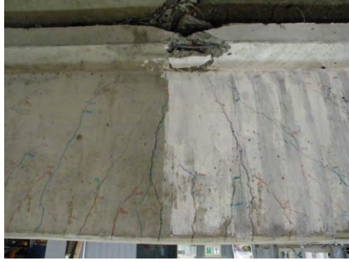
Figure 6.1: Specimen T.6.18.6.S at failure (flexural)
