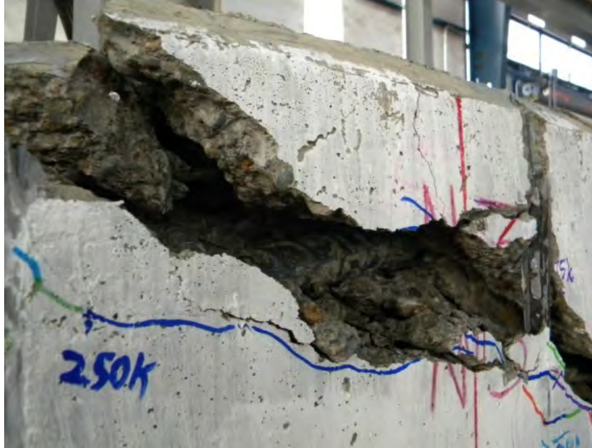
Figure 6.13: Specimen IT.7.18.12.S detachment of concrete cover between grid lines N1 and N3
