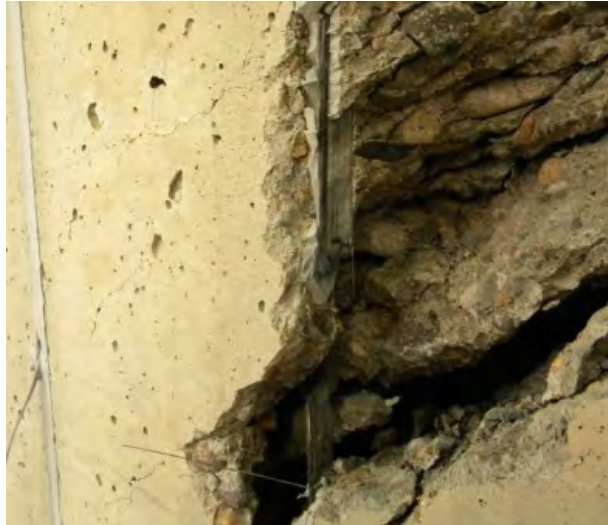
Figure 6.20: Rupture of CFRP strip without slip relative to surrounding epoxy or concrete
