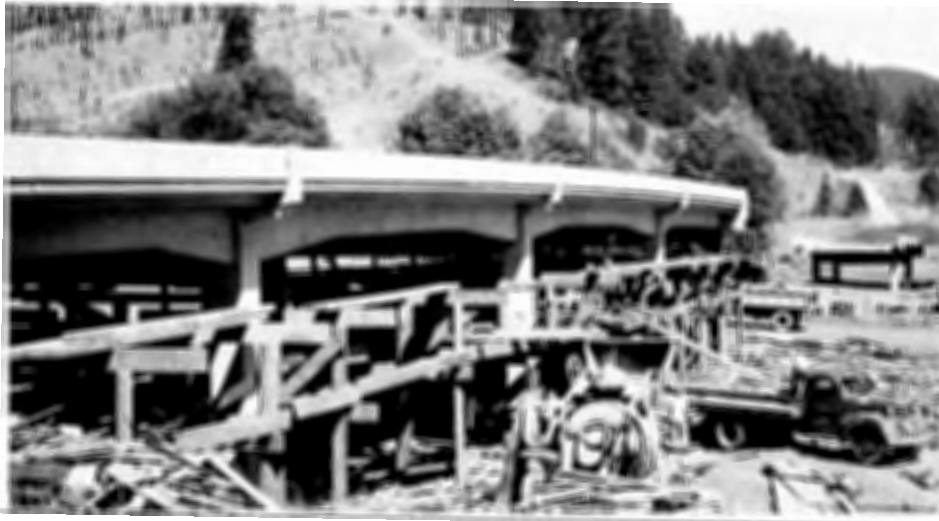
Figure 2.19. Haunched Cast-in-Place Beams, Pacific Highway (I-5) Overpass at Anlauf-Elkhead, Lane County, Bridge #2594, July 1953 Source: ODOT Bridge Files
