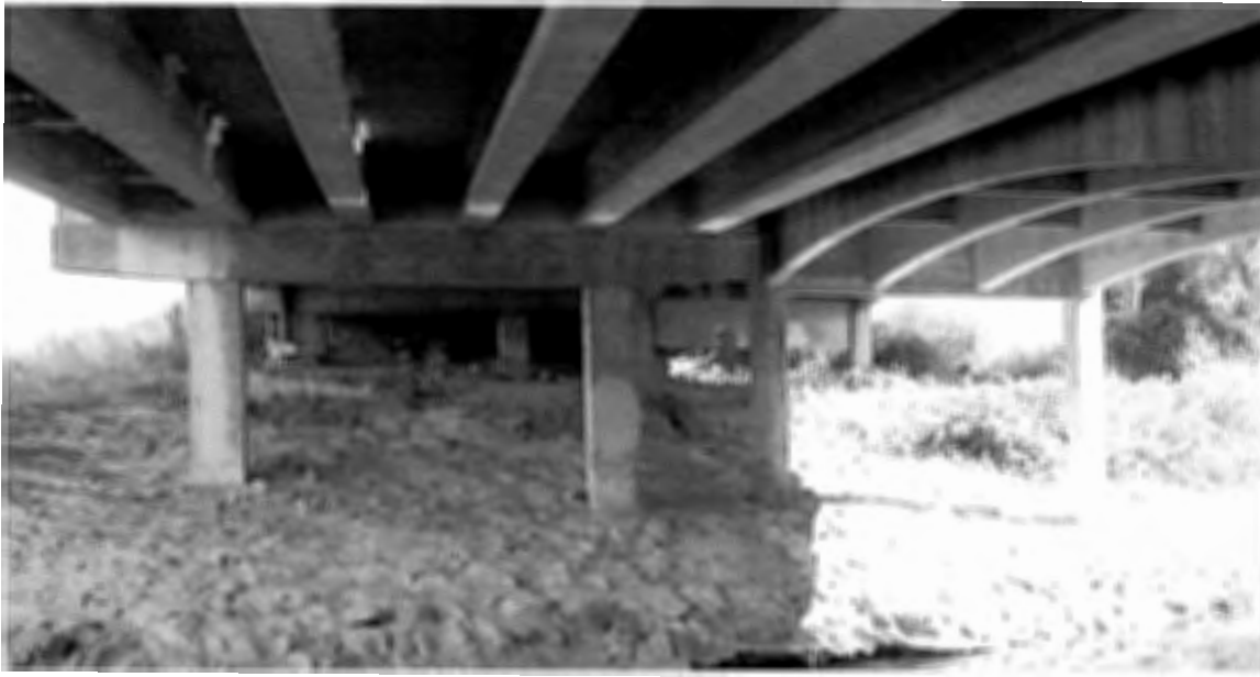
Figure 2.26. Isaac Constant Bridge #697, Central Point, Oregon showing two different variants of square section support piers. (Note pre-stressed I-Beam girders on left, haunched, cast-in-place girders on right.) Source: Author Photograph, November 2002
