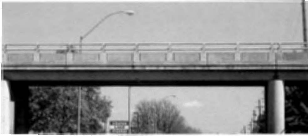
Figure 2.11. "Two Pipe" Variant, Rail Type C/D Medco Lumber Haul Road/Biddle Road Overpass, Jackson County, Oregon Source: Author Photograph, May 2003
