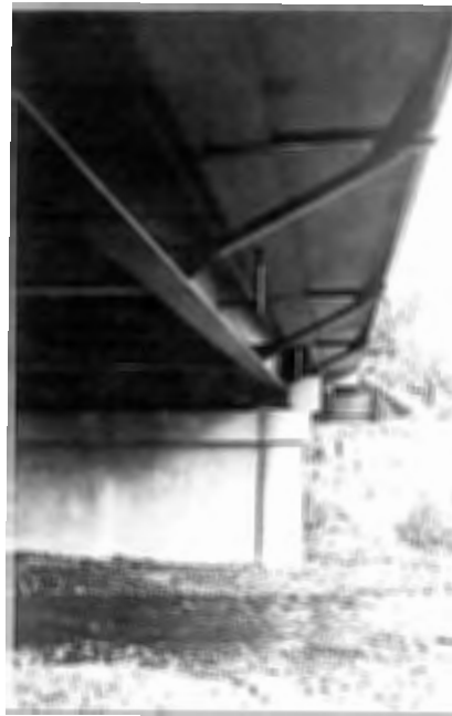
Figure 2.28. "Barbell" Type Piers Supporting a Rolled Steel Beam Bridge with Cantilevered Sidewalks. Benke Bridge, Nehalem Hwy, c1934 Source: ODOT Archive
