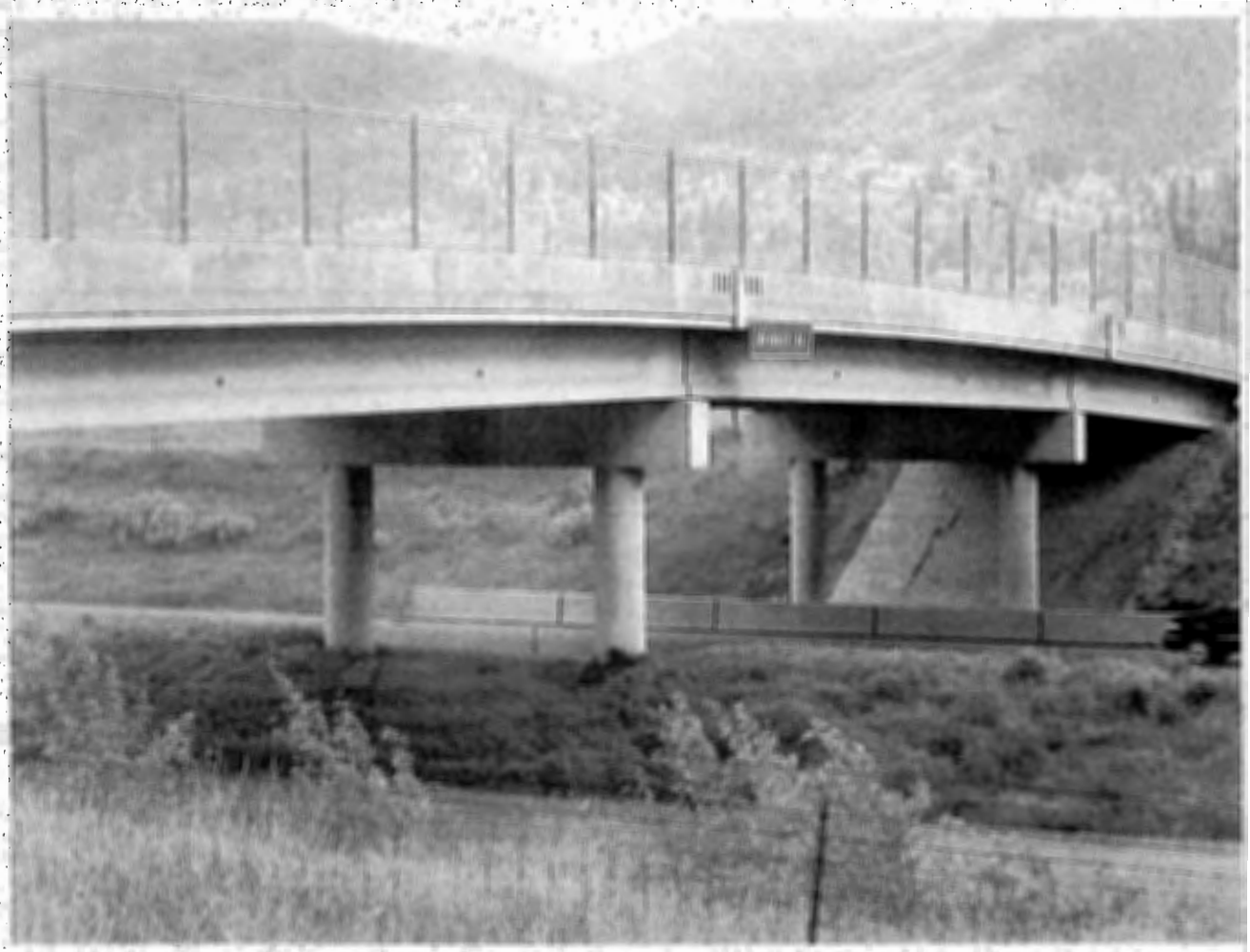
BRIDGE No. 8739, MOUNTAIN AVE OVER INTERSTATE 5, ASHLAND, JACKSON COUNTY OREGON, LOOKING SOUTH 259-Foot long Precast Concrete Girders (1963) with Type A/B Bridge Rail, Modified with Protective Fencing June 2003
