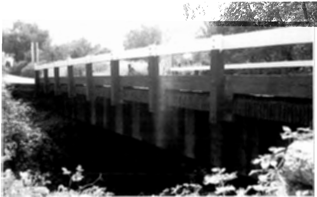
Figure 1.5. Bridge 29C77, Rapp Road at Wagner Creek (Jackson County Bridge No. 57) Timber, Stringer/Multi-Beam Girder (OBI Code #702), 46 feet long, built 1955 Source: Author Photograph, August 2003
