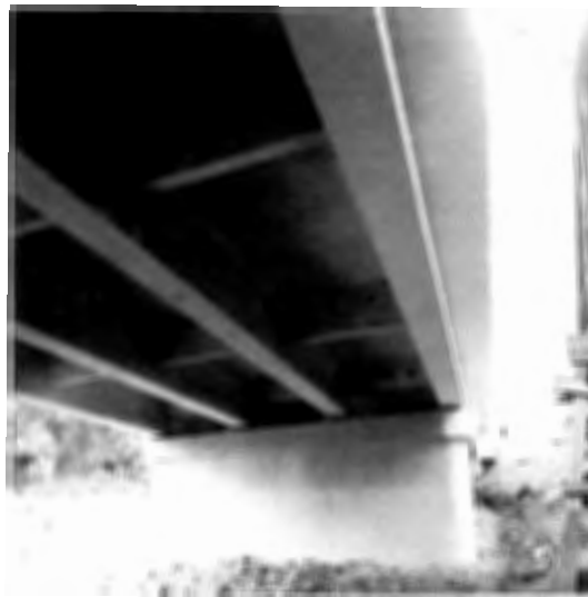
Figure 2.29. Flat Panel Concrete Pier, Pudding River and Butte Creek Overflow, 1970 Source: ODOT Archive
