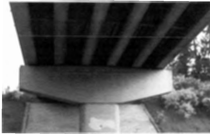
Figure 2.30. Various Monolithic Concrete Bridge Pier Designs Interstate-5 Examples Source: Author Photographs, May 2002
