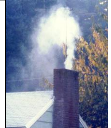
Excessive smoke is a sign your stove is burning inefficiently.
